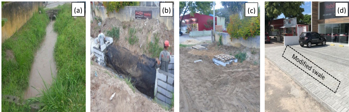
Figure 1 (a) Infiltration swale before modification, (b) Modification and construction of a drainage bedding made with chitin, (c) Modified swale in final stages of completion, and (d) Modified swale completed and sidewalk paving finished.
